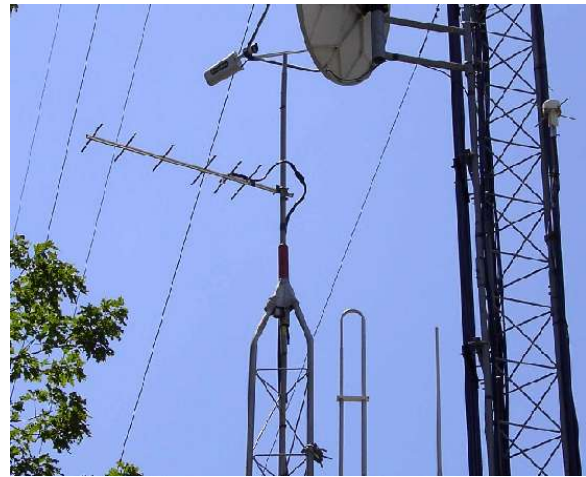
Grand Rapids Link Receiving Antenna, 5-Mile Hill
